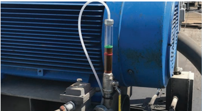
Vent Tube Option - Cooling Tower
