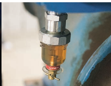
Large Blower - Wastewater Treatment Plant
