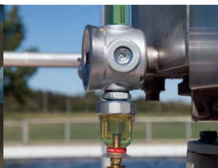
Clarifier - Wastewater Treatment Plant
