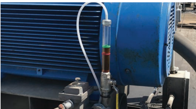
Vent Tube Option - Cooling Tower
