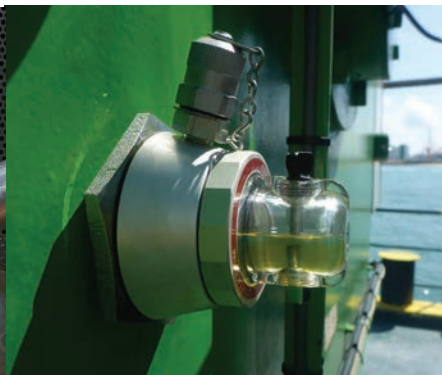
Mooring Winch - Ocean Dredger
